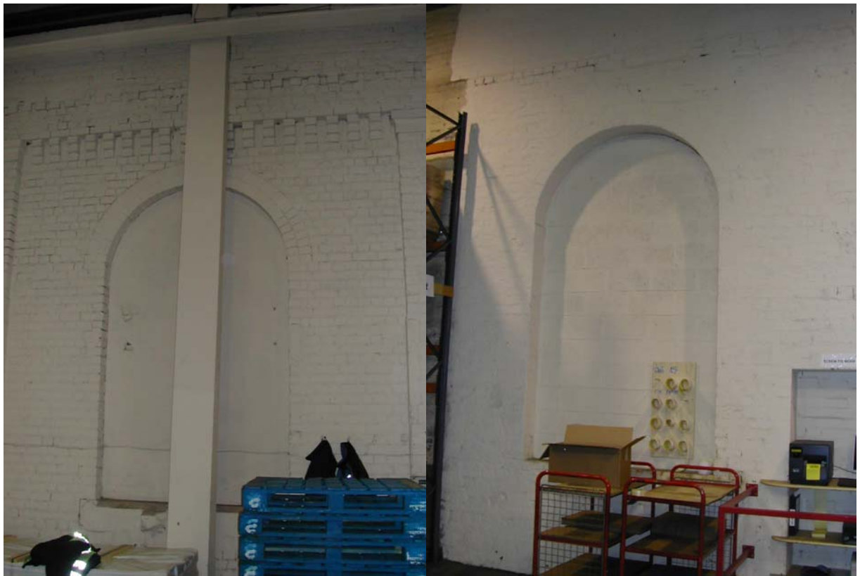
Loco shed window opening and eaves corbelling from outside (left) and inside (right).
