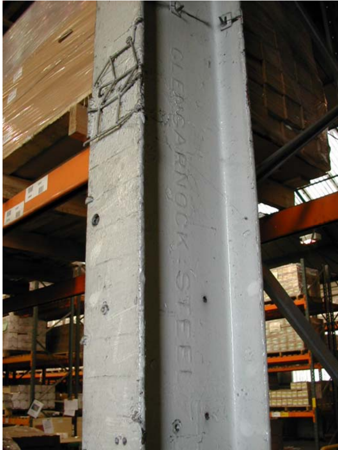
A stanchion between bays 1 and 2. The Glengarnock Steel Co. Ltd. was trading from 1890 to 1915, the works being taken over by Colvilles Ltd. then British Steel.
