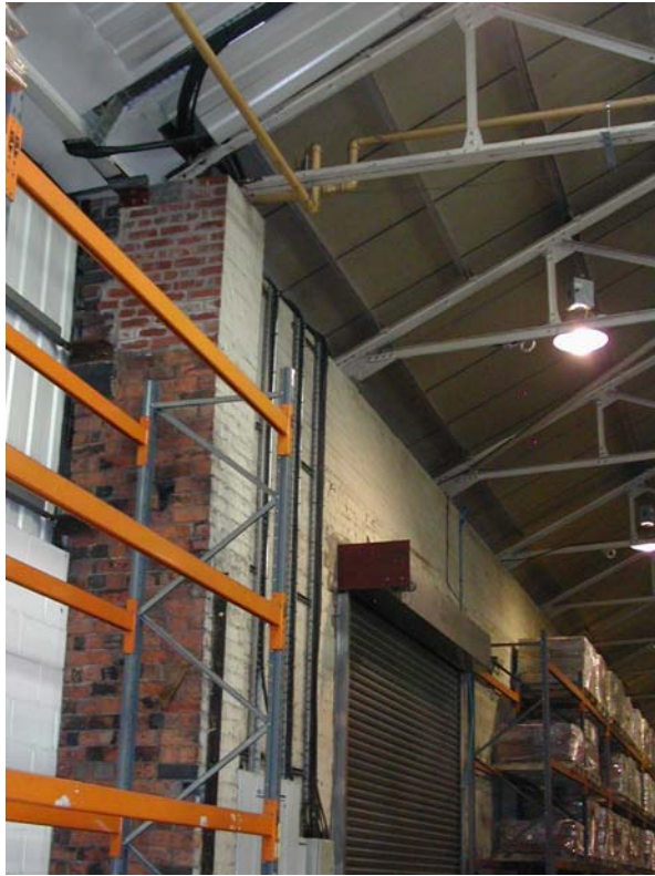
South-west end of loco shed, as altered for 1939 re-roofing (and again recently?), showing unpainted brick pier.
