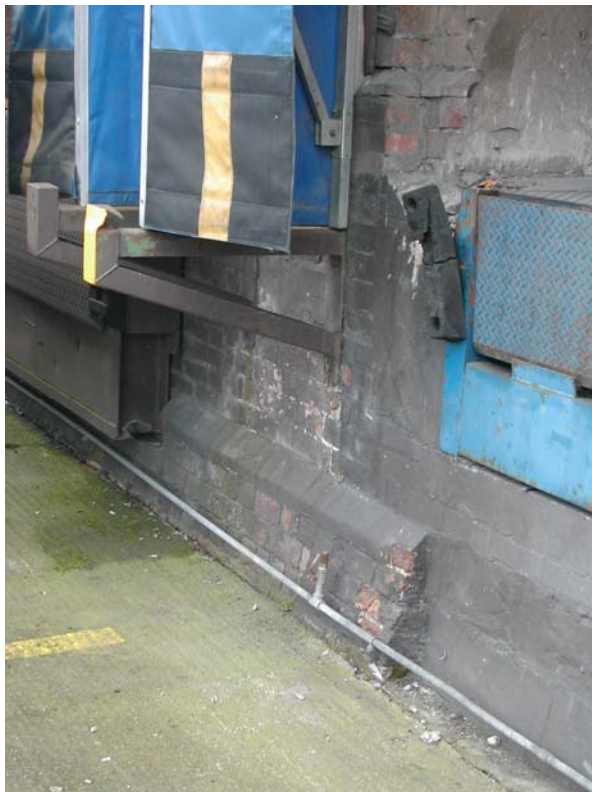
North-east end of loco shed, showing original openings adapted for lorry loading, and battered plinth.
